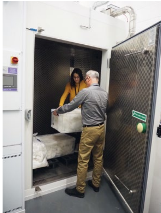
FIGURE 6. In addition to inspection and quarantine spaces, the pest treatment facility in the WCEC building includes a walk-in freezer. Photo: Trustees of the British Museum.
