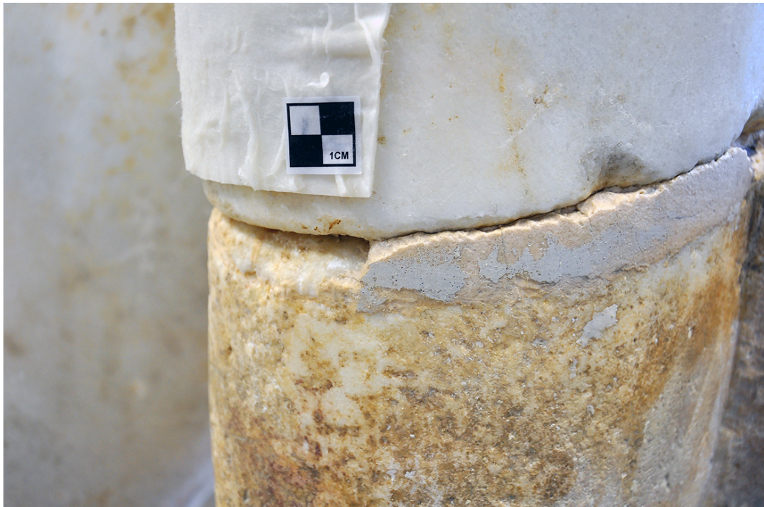
Detail of the left leg during the removal of the plaster and cement (Sorel?) sealing
